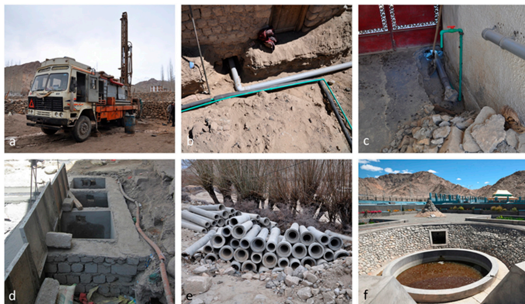
a Well driller, b Newly laid household water supply and sewage pipelines, c Water access on private premises, d Septic tank, e Stored pipelines for the UIDSSMT scheme, f Faecal Sludge Treatment Plant (FSTP)
